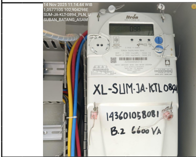
Picture 2.1.3 - Stand Meter Before Upgrade
