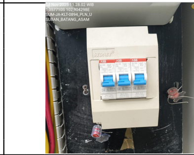
Picture 2.1.2 - MCB KWH Meter After Upgrade
