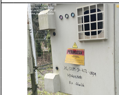
Picture 2.1.7 - KWH Panel Closed Door Condition
